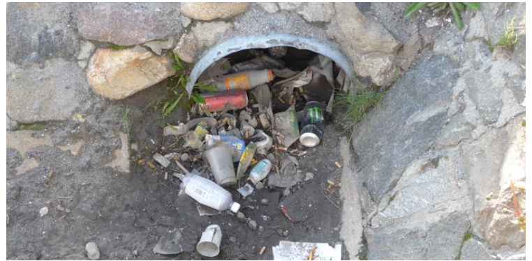
Driveway Culvert Blocked with Debris
