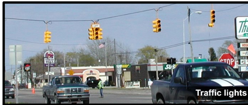
Figure D-1: Example of traffic signals
