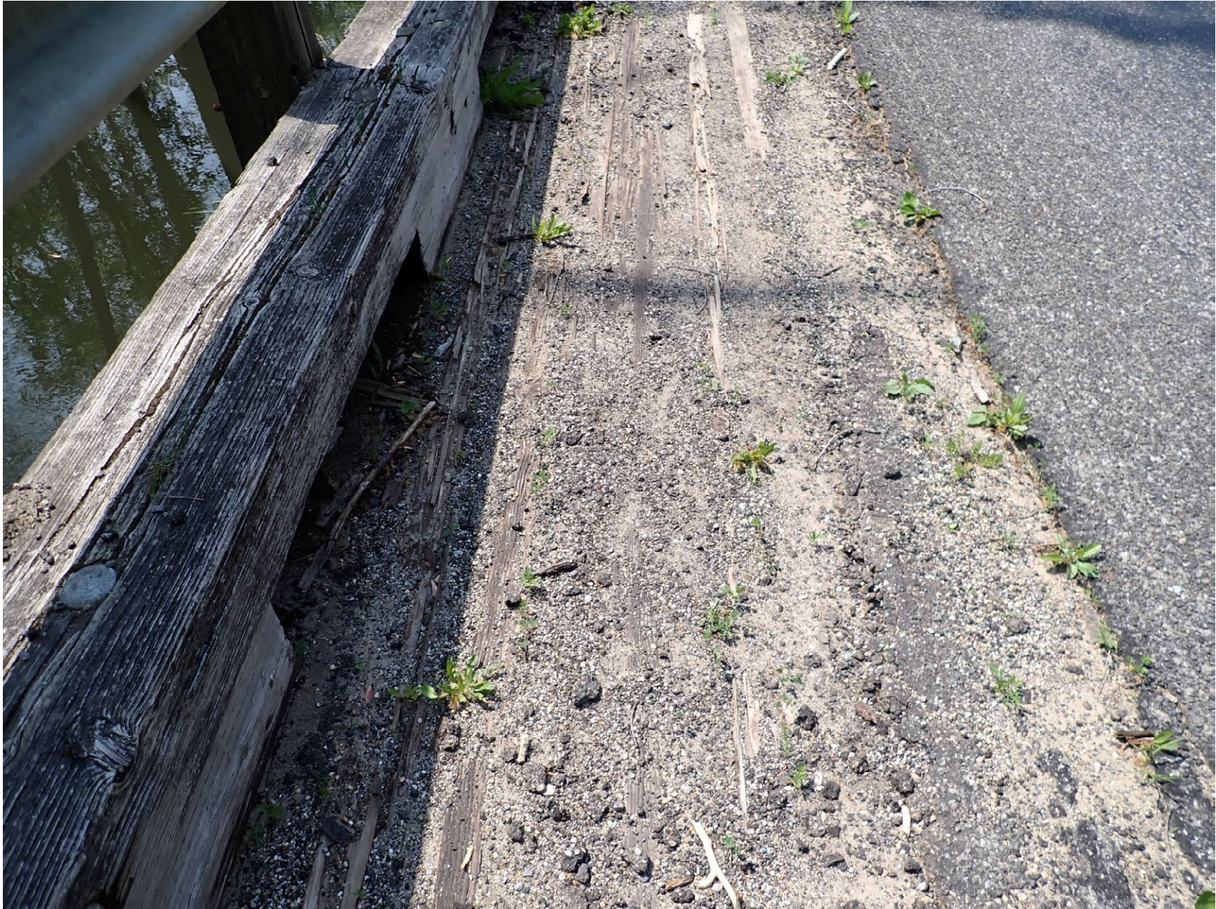
Deck boards exposed along edges, rotting; vegetation growing in edges
