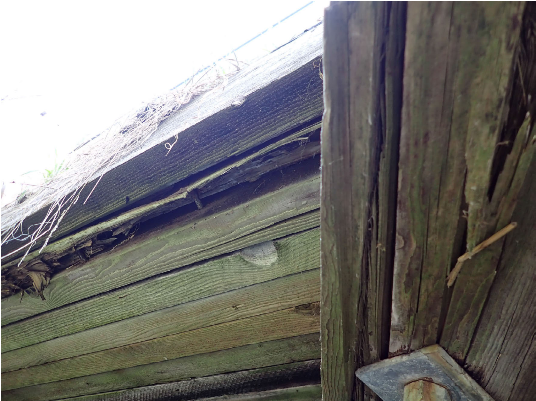
West end of span 1S: Spreader beam damaged, west fascia board and board 2W rotting
