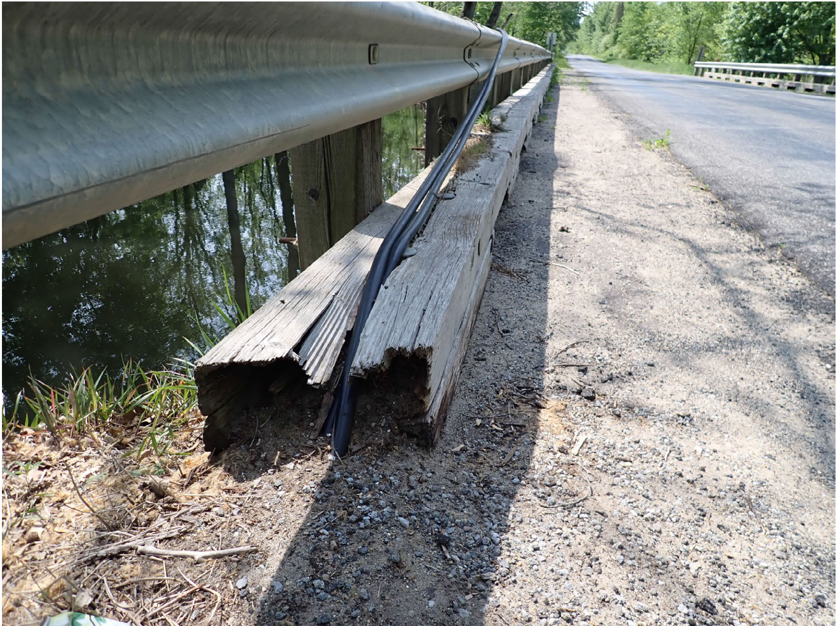
Brush block rotting with vegetation growing out of it
