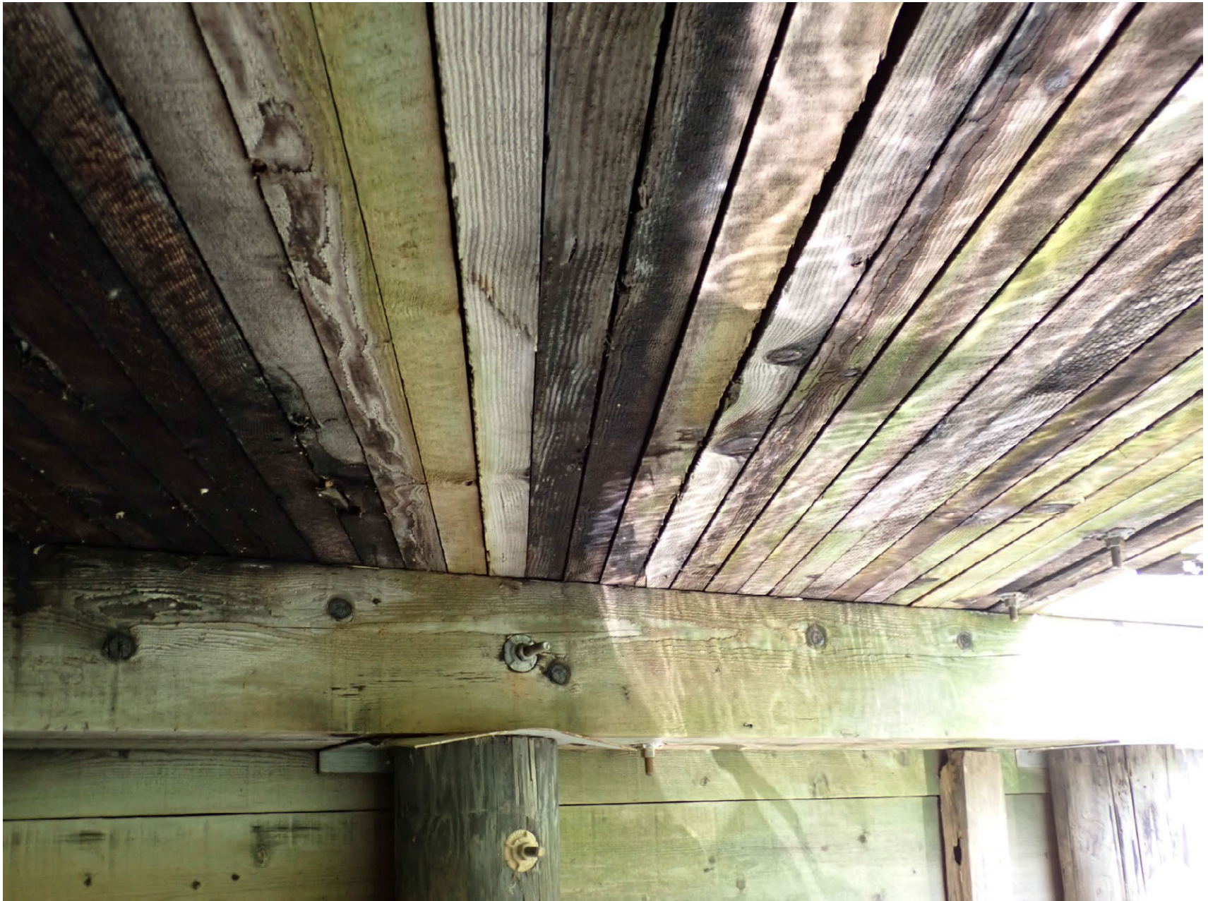
Typical cracked deck board
