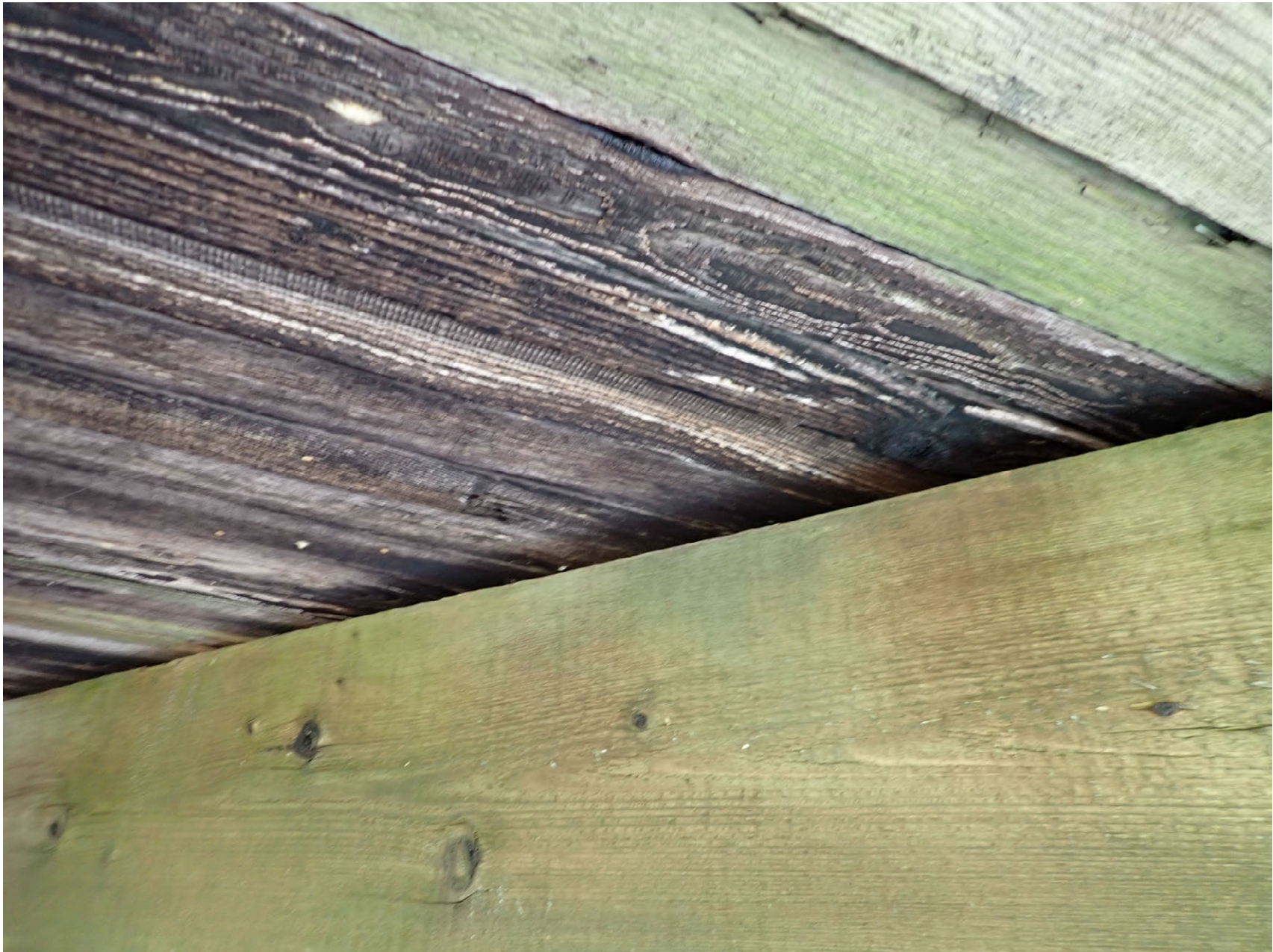
Typical gaps between deck boards and spreader beams
