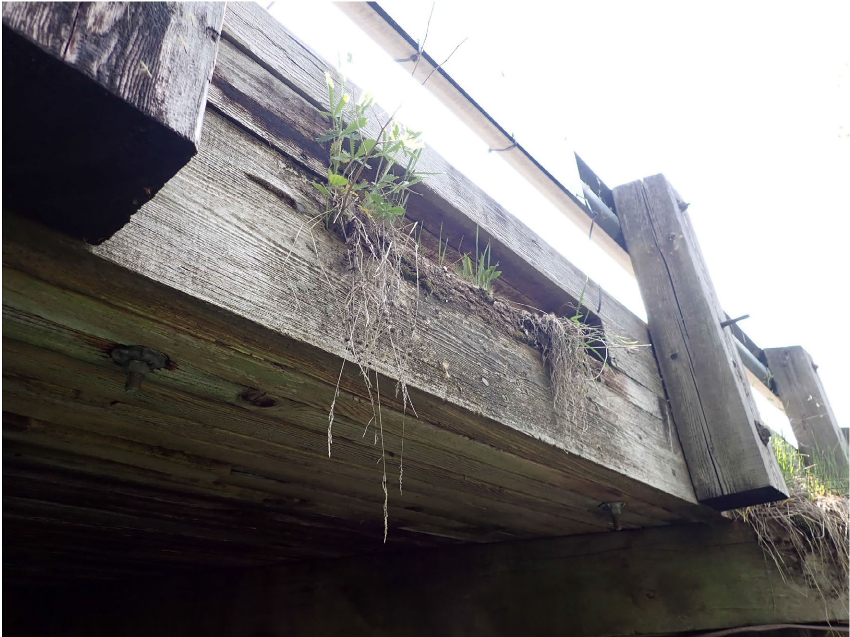
West fascia board rotting
