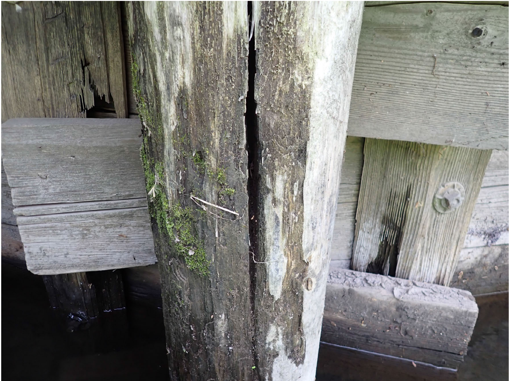
Vertical split and rot in south abutment pile 1W
