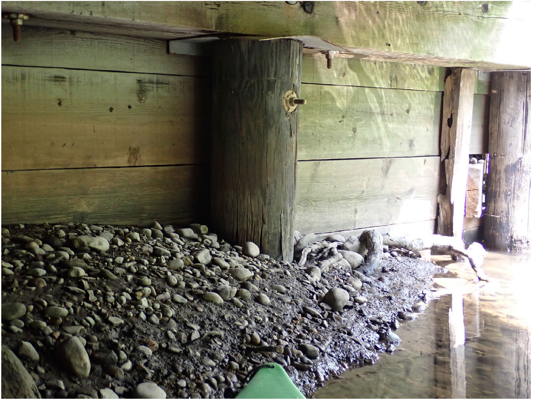
North abutment pile brooming
