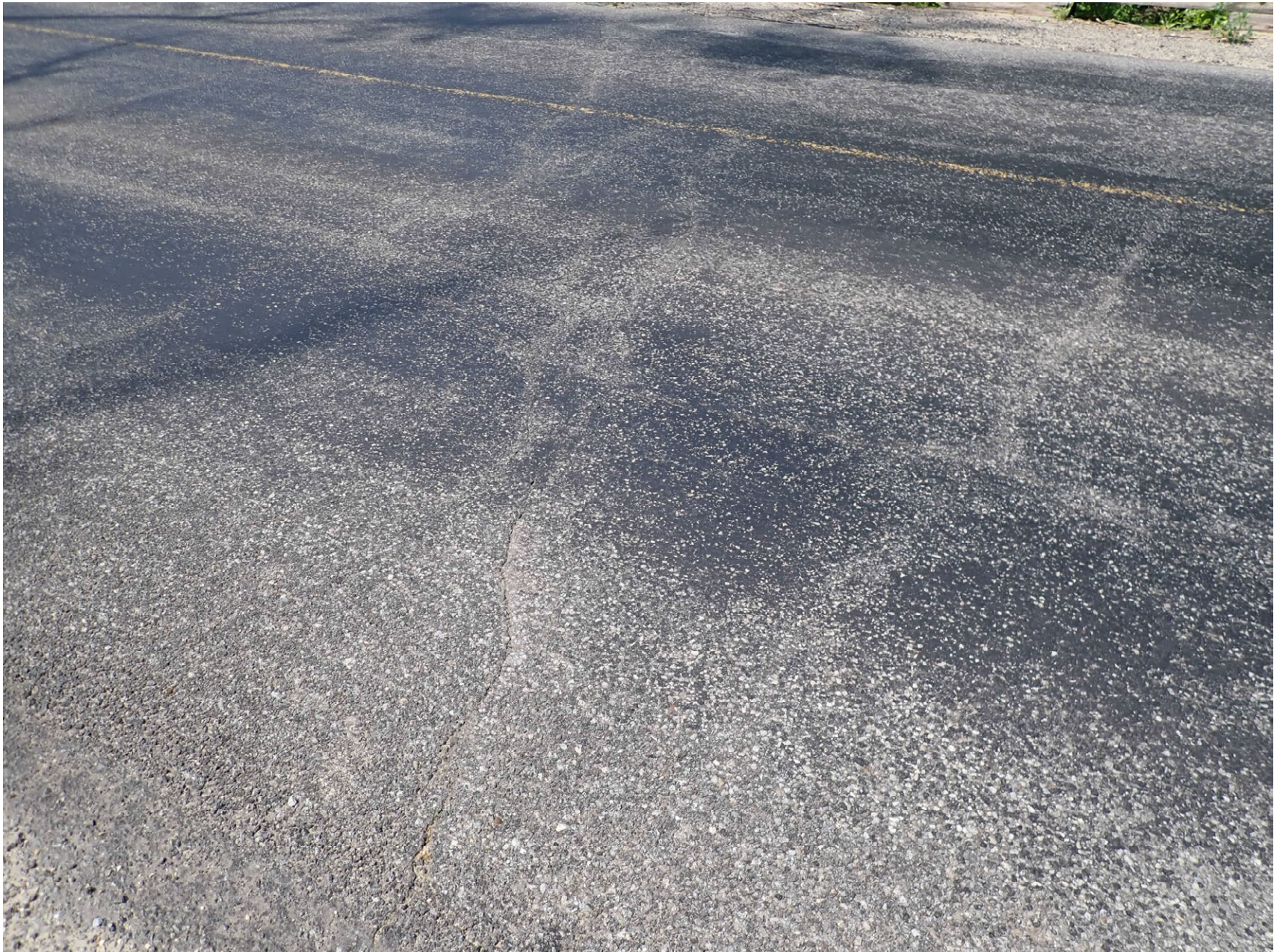
HMA cracked over piers; transverse and longitudinal reflective cracking
