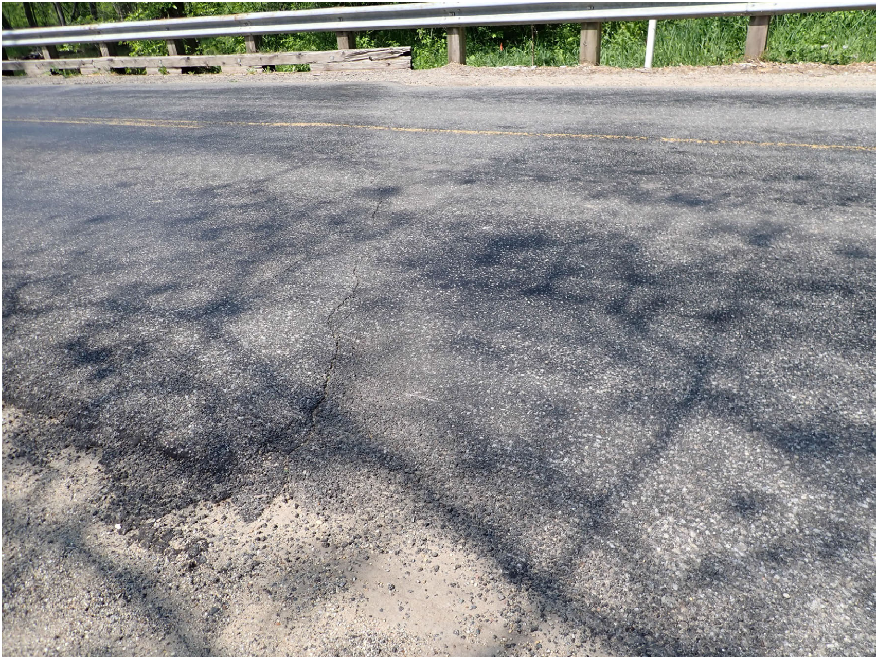
HMA cracked at reference lines
