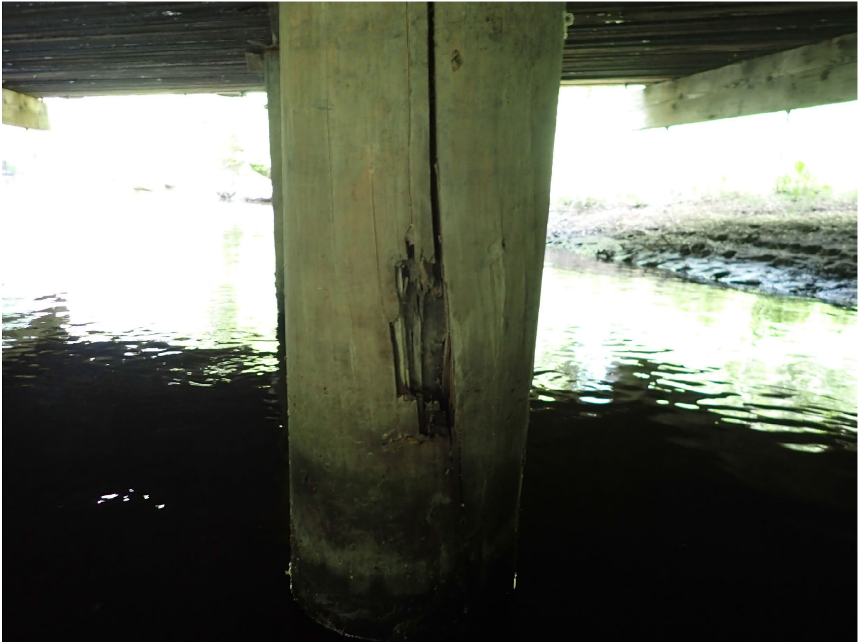
Split and damage in pier pile
