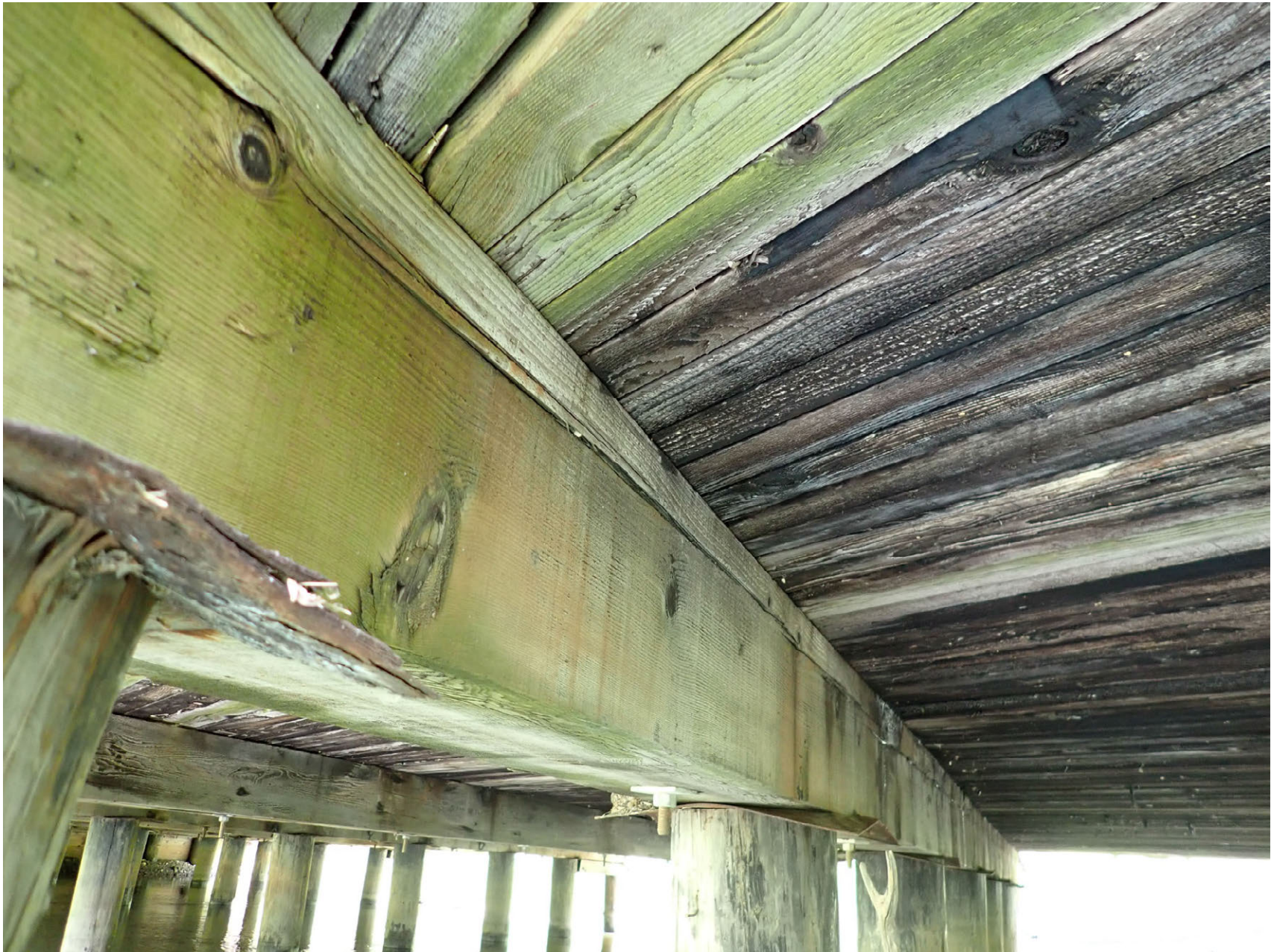
Typical pier cap crushing (pier 4N shown)
