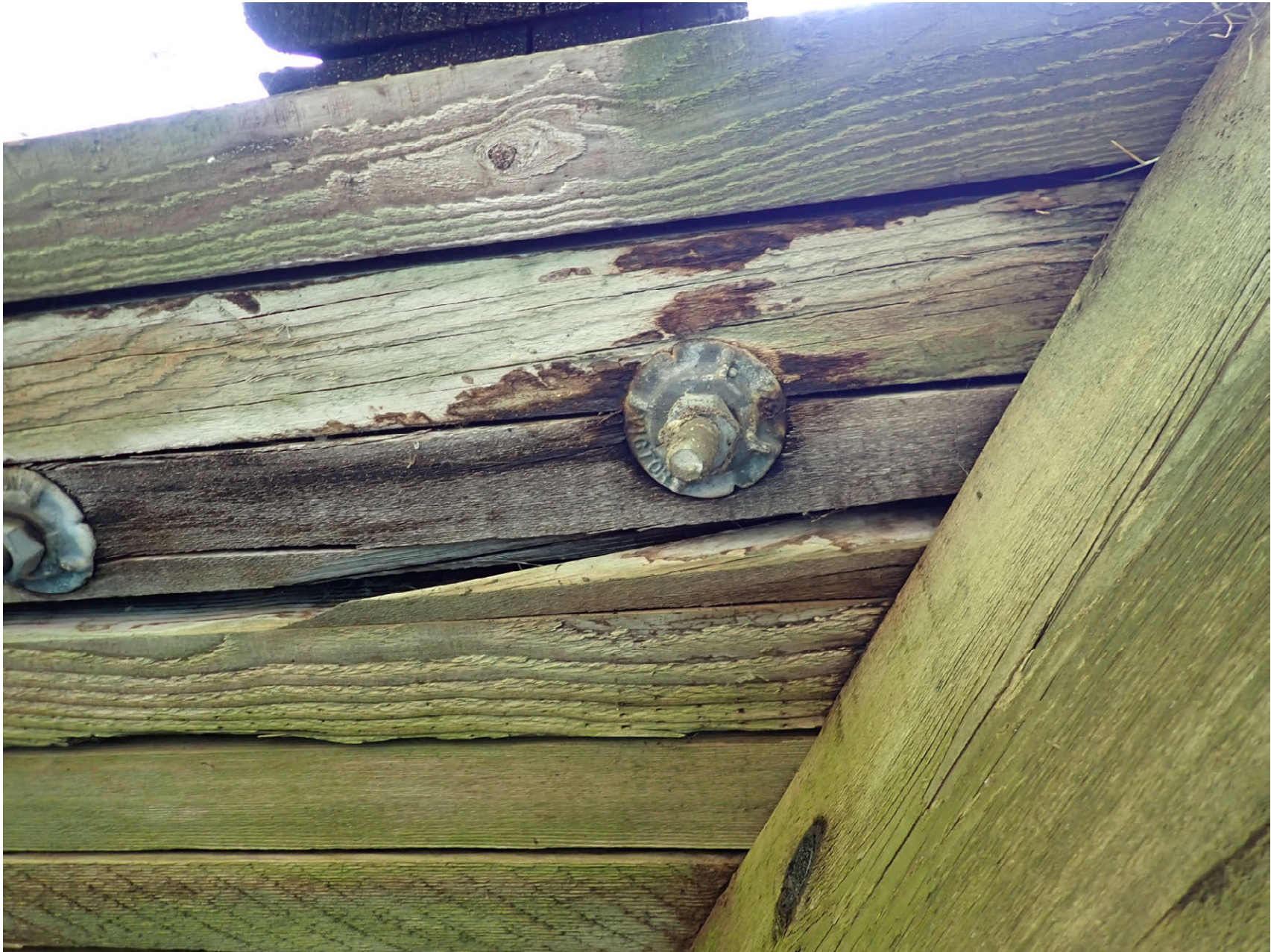
Deck board cracked and starting to rot near fascias
